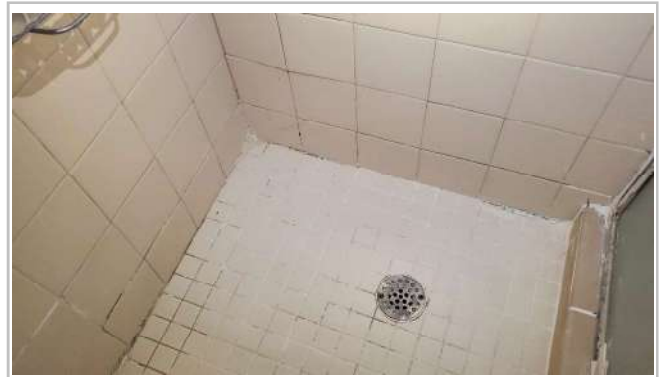
Bathroom # 4 shower needs to be resealed. Repair as needed.
