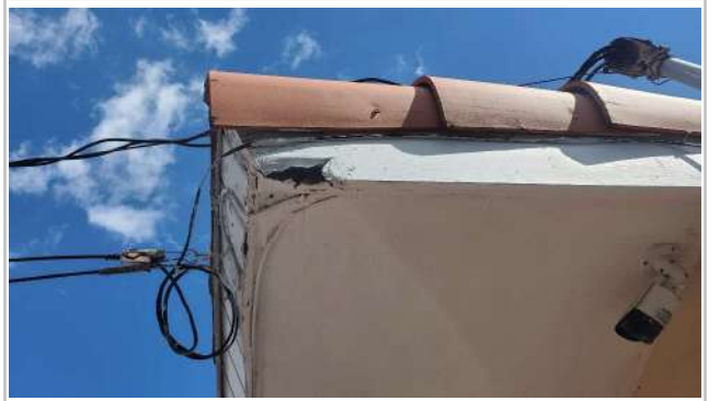
Fascia Board throughout the home has wood rot. Replace as needed.
