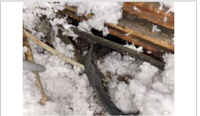
Cloths wires were found in attic with live power. Replace as needed.
