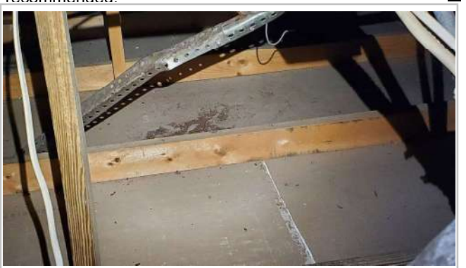
Found termite droppings and wings in garage attic. Termite tent recommended.
