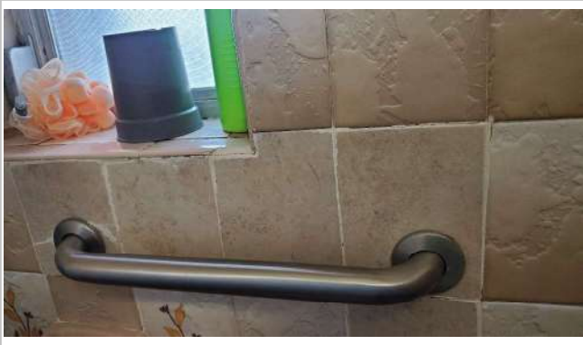
Bathroom # 2 has 3 cracked tiles in the wall. Replace as needed.
