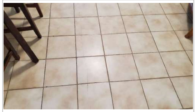
Dining/ living/ family room has over 20 cracked tiles. Replace as needed.
