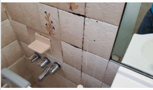
Bathroom # 2 shower needs to be resealed. Repair as needed.
