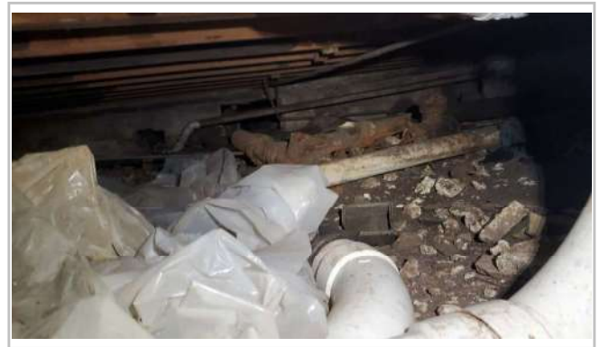
Crawl space cast iron pipes debris left overs view.
