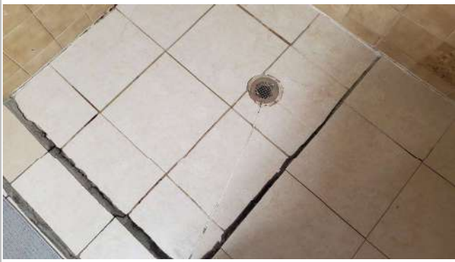
Master bathroom shower floor has 5 cracked tiles. Replace as needed.
