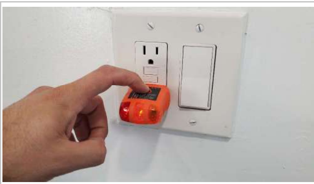
Bathroom # 3 GFCI outlet is not tripping. Replace as needed.
