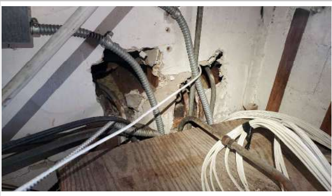
Attic has hole. Wild life and moisture could come in. Repair as needed. Pest control recommended.
