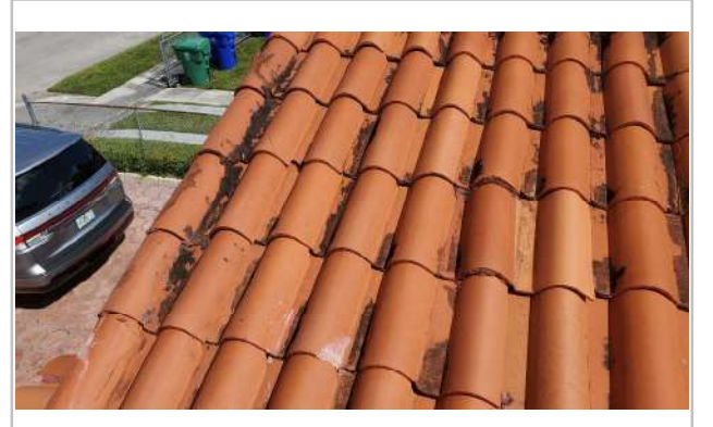
Concrete roof has 15 or more cracked tiles. Repair/replace as needed.
