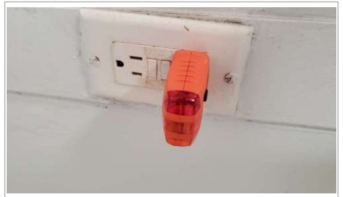
Master bathroom GFCI outlet is not working. Repair/replace as needed.
