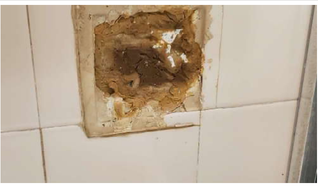
Bathroom # 4 soap holder is missing. Replace as needed.
