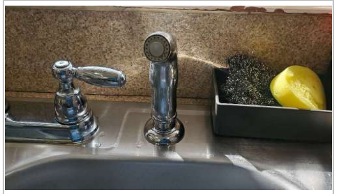
Kitchen faucet hose sprayer is not working. Repair/replace as needed.
