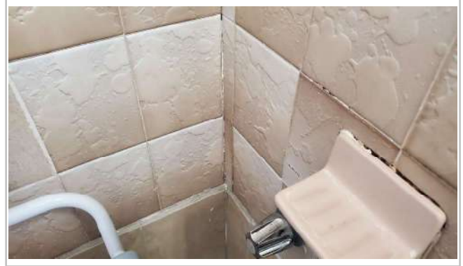
Bathroom # 2 shower needs to be resealed. Repair as needed.
