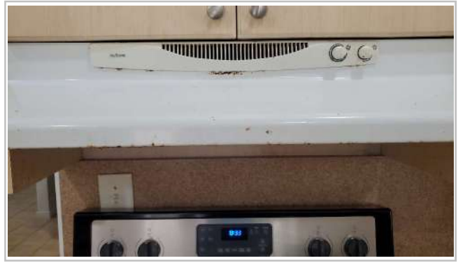
Kitchen exhaust panel is rusted.
