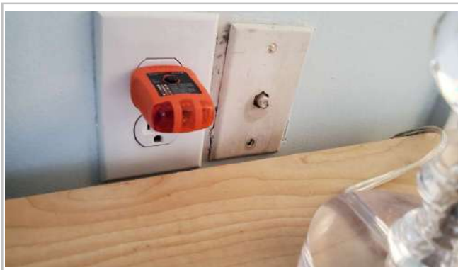
Living room # 2 outlet has no power. Repair/replace as needed.
