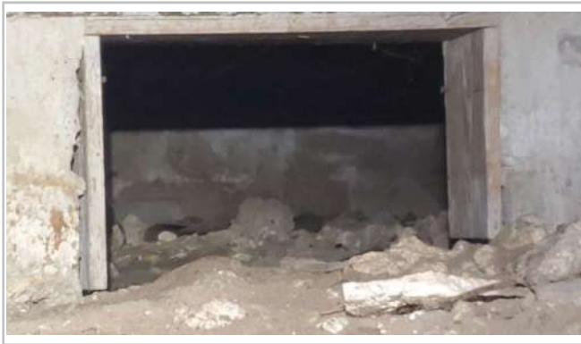
Crawl space debris left overs view.
