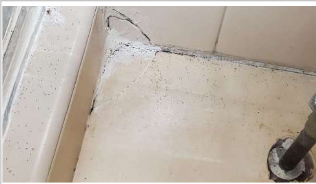
Bathroom #4 floor near toilet has termite droppings. Termite tent recommended.
