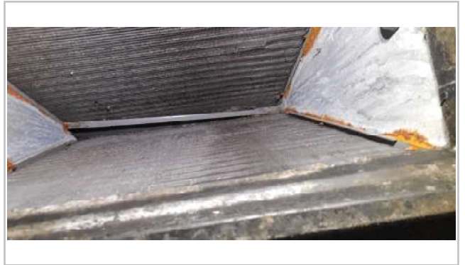
A/C air handler # 2 needs acid wash and flush. Repair as needed.
