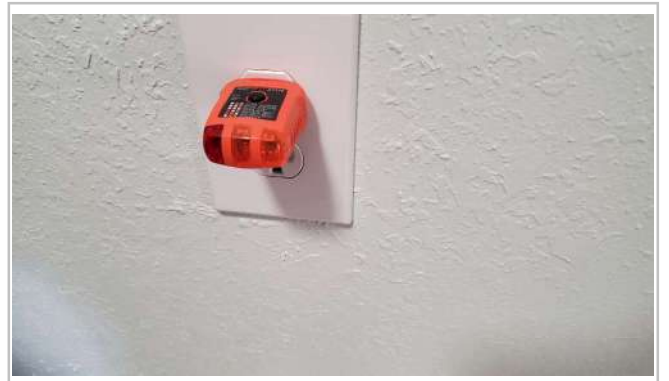
Dining room outlet has no power. Repair/replace as needed.
