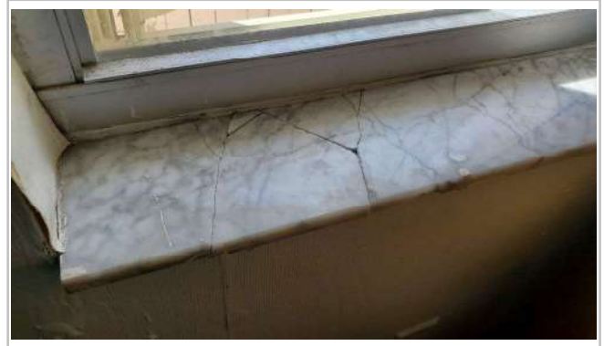
Living room #2 window sill is damaged. Replace as needed.
