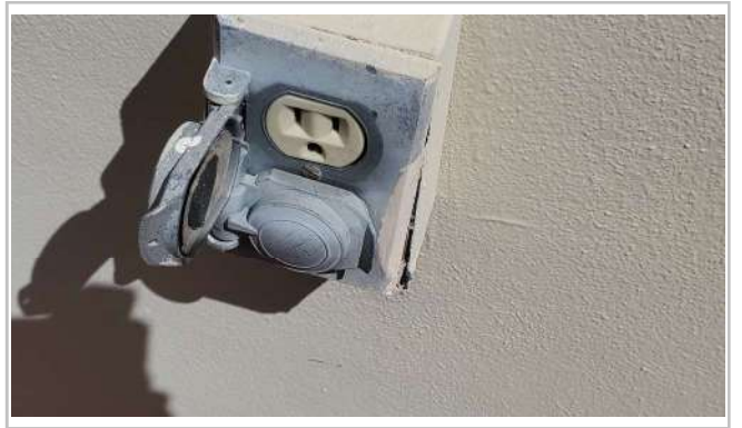
Rear outside electrical outlet needs to be GFCI. Replace as needed.
