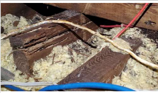
House main attic has wood rot due to termites. Termite tent recommended.
