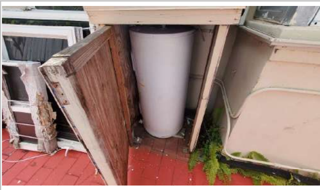
Water heater is outside the home, has a shed but is still exposed to the weather. Replace in the near future.
