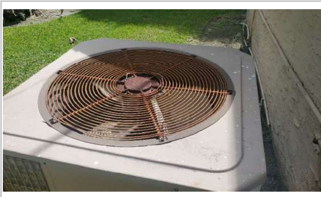
A/C air condenser exterior coil is damaged in the bottom. Replace as needed.
