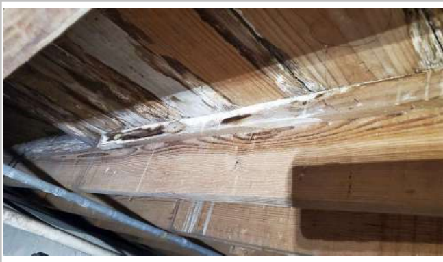
Crawl space underneath wood has wood rot and water stains. Repair/replace as needed.
