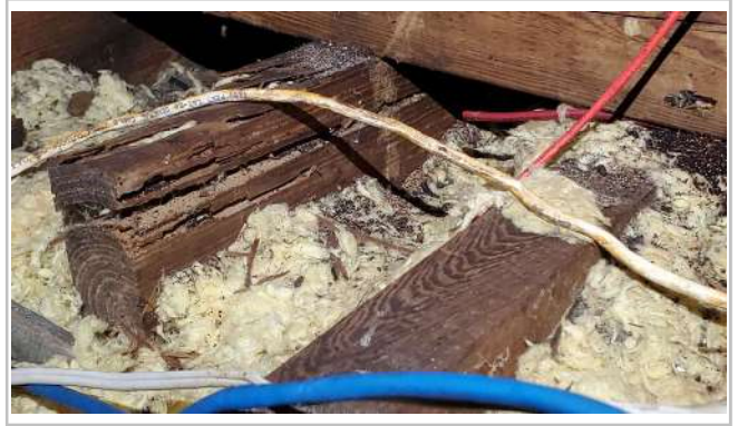
Cloths wires were found in attic with live power. Replace as needed.
