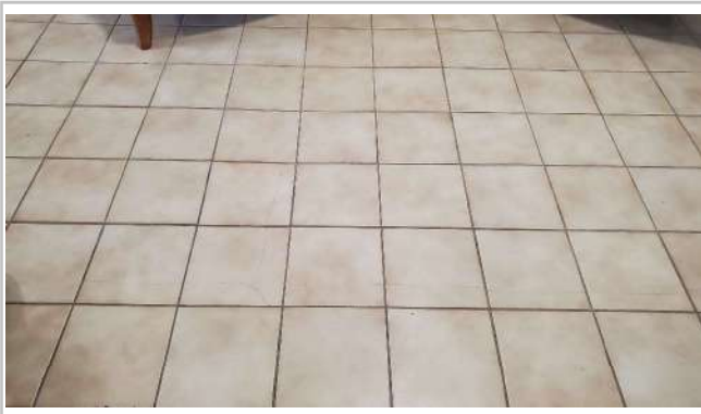
Dining/ living/ family room has over 20 cracked tiles. Replace as needed.
