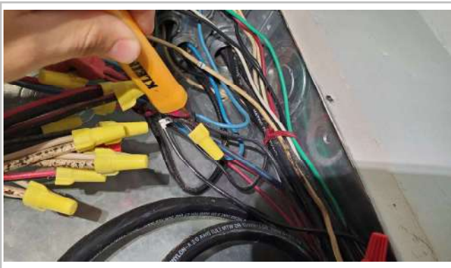
Electrical panel has cloth wires. Replaces as needed.
