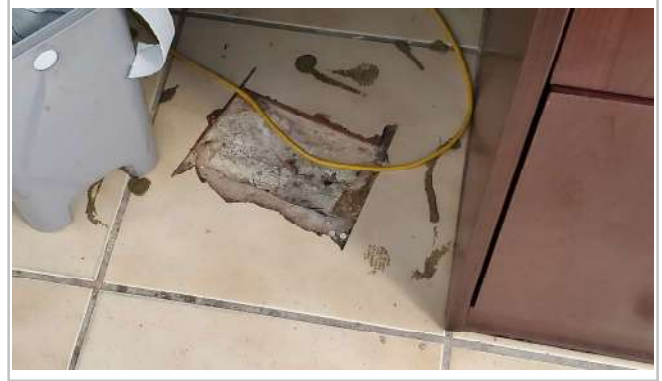
Garage floor is damaged under office area. Replace as needed.
