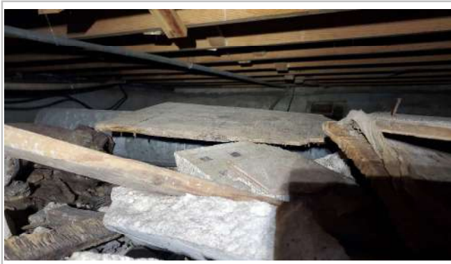
Crawl space debris left overs view.
