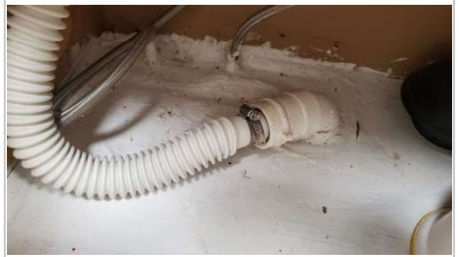
Master bathroom cabinet under sink is damaged. Replace as needed.
