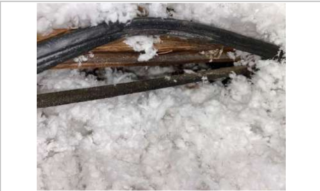
Cloths wires were found in attic with live power. Replace as needed.
