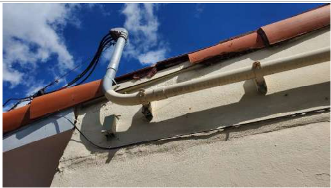
Right side roof tiles are missing. Replace as needed.
