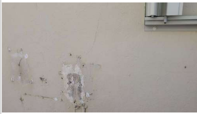
Right side outside wall has a stress crack. Repair a needed.
