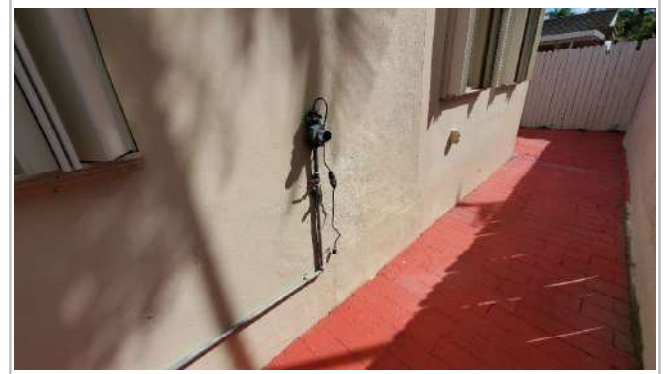
House use to have gas lines and were left behind. Remove as needed.
