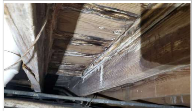
Crawl space underneath wood has wood rot and water stains. Repair/replace as needed.
