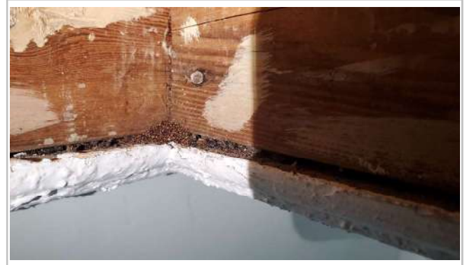
Found termite droppings and wings in main house attic. Termite tent recommended.
