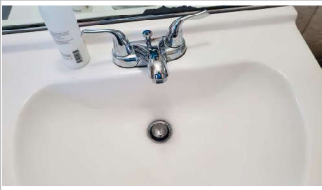
Bathroom # 2 sink manual drain stopper is damaged. Replace as needed.
