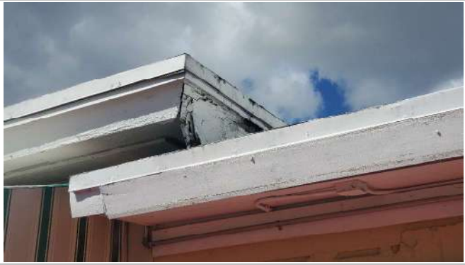
Fascia Board throughout the home has wood rot. Replace as needed.
