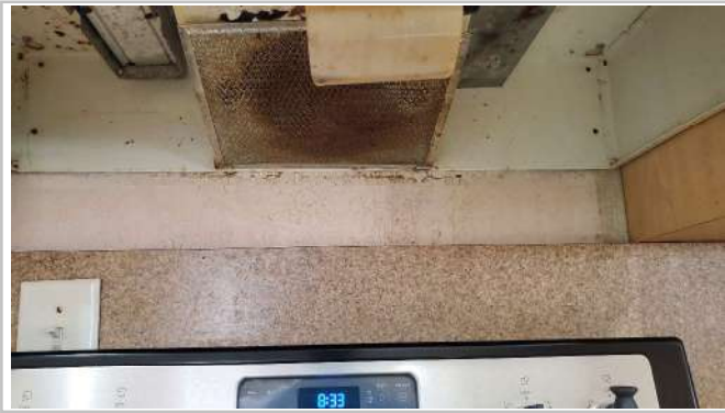
Kitchen exhaust fan filter is dirty. Replace as needed.
