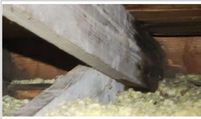
Attic beam has wood rot from previous leak. Repair/replace as needed.
