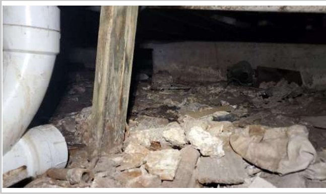
Crawl space debris left overs view.
