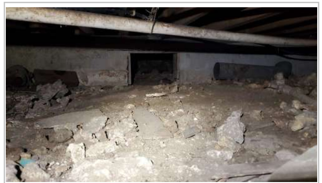
Crawl space debris left overs view.
