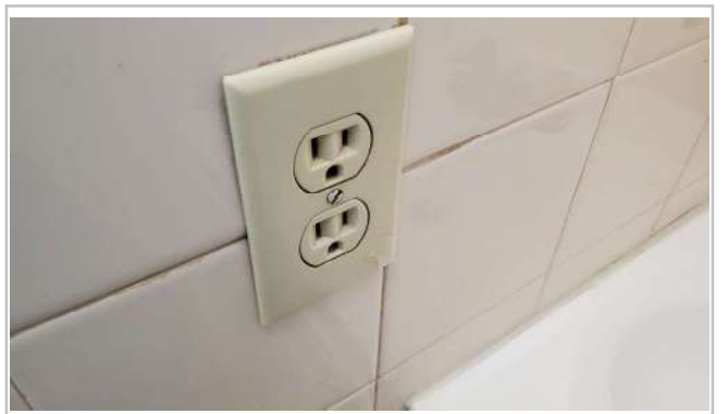
Bathroom # 4 outlet needs to be GFCI. Replace as needed.
