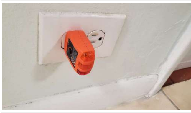
Master bedroom outlet has no power. Repair/replace as needed.
