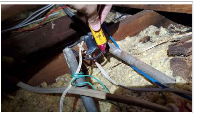
Cloth wires found in the attic with power. Replace as needed.
