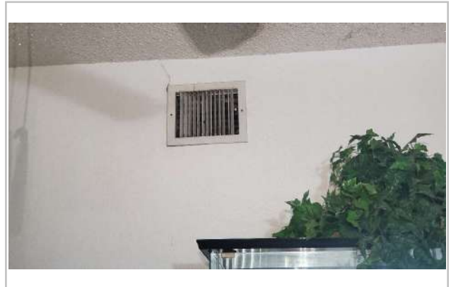
A/C air ducts need to be clean/repair/replaced, mold like substance found throughout the home walls. There was a
