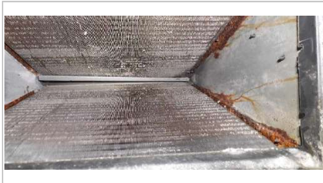
A/C air handler # 1 needs acid wash and flush. Repair as needed.
