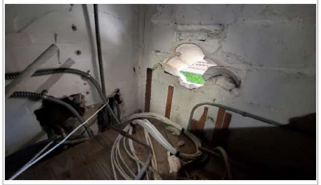
Attic ceiling has hole leading to outside. Wild life and moisture could come in. Repair as needed. Pest control recommended.
