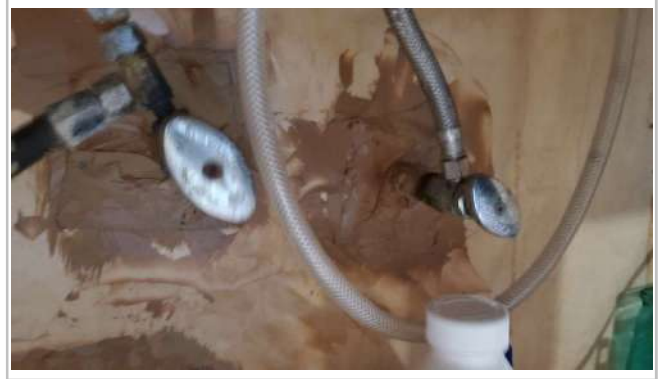
Kitchen cabinet is damaged near shut off valves. Replace as needed.
