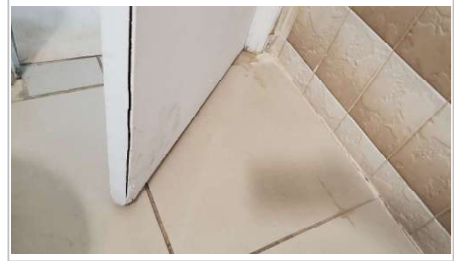
Bathroom # 3 door is damaged in the bottom. Replace as needed.
