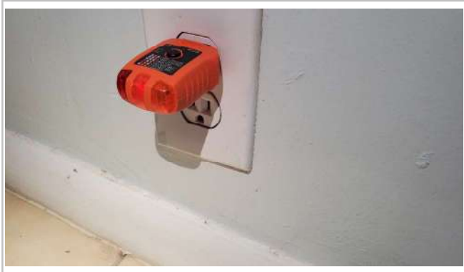
Bedroom # 3 outlet has no power. Repair/replace as needed.
