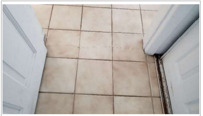
Bedroom #4 has 3 cracked tiles. Replace as needed.
