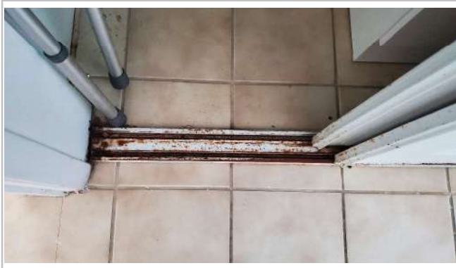
Bedroom #4 sliding closet door rail is rusted. Replace as needed.
