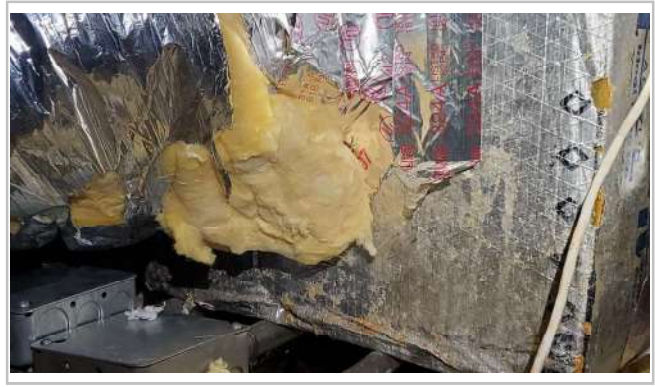
Garage attic air duct is torn. Replace as needed.
