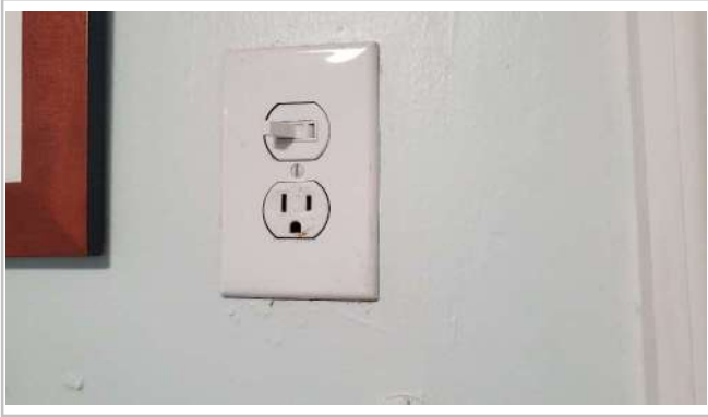
Garage outlet has no power. Repair as needed.
