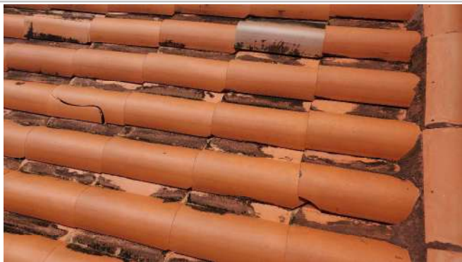
Concrete roof has 15 or more cracked tiles. Repair/replace as needed.
