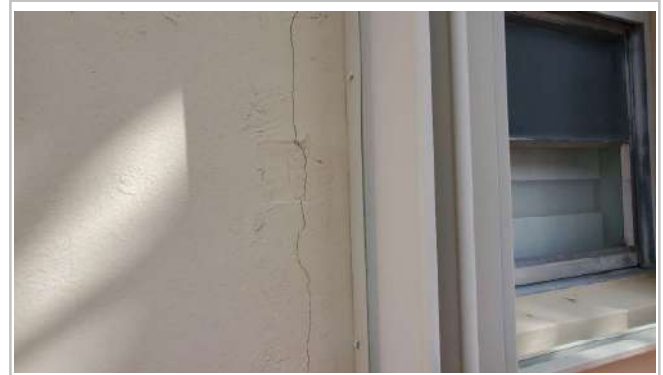
Large settlement crack found at right outside wall running vertical. Evaluation and repair by qualified licensed contractor for appropriate estimate recommended. +
