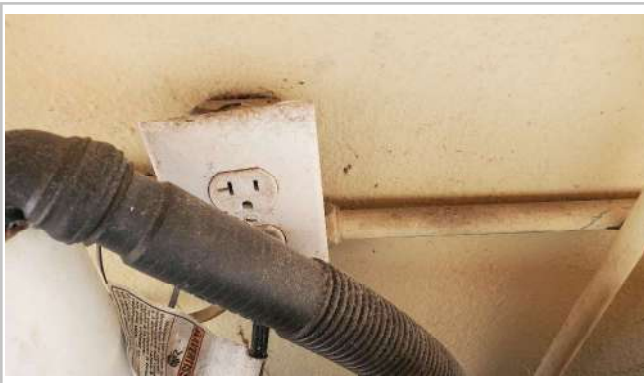
Rear outside electrical outlet needs to be GFCI and needs water proof cover. Replace as needed.
